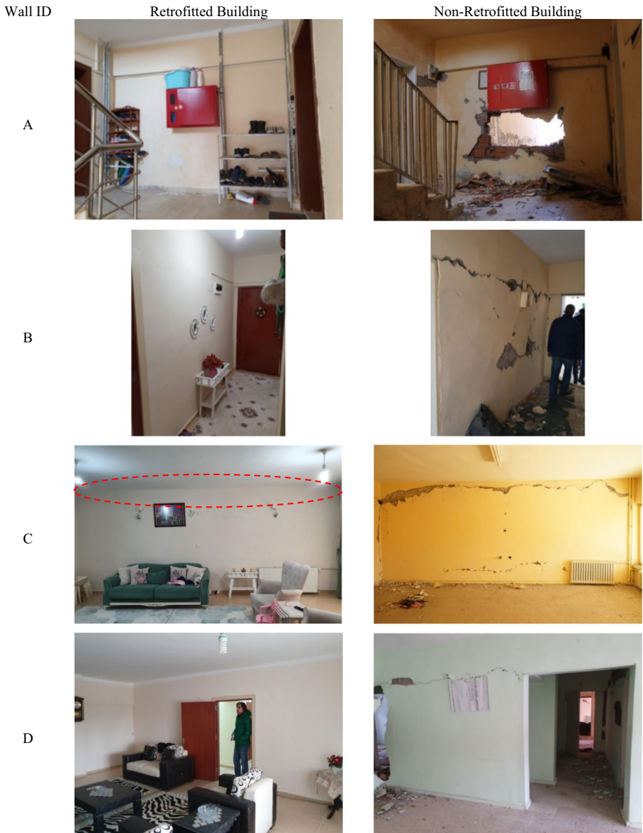
Fig. 6 Damage of the retrofitted and non-retrofitted buildings
