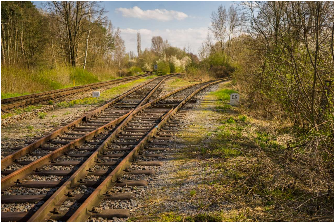
Image 8 - another view of the switch with a distance marker of the branch line on the right
