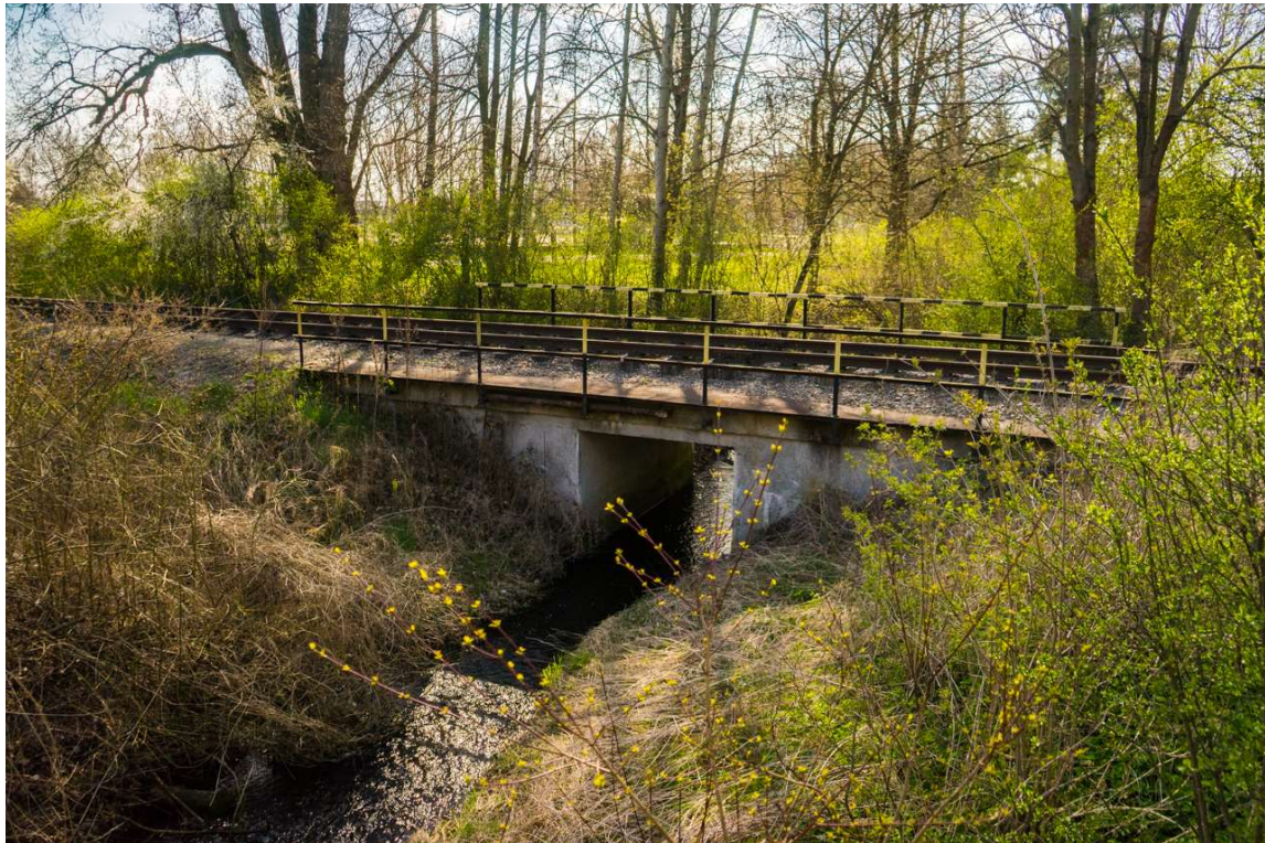
Image 9 - concrete beam bridge located on the main track of the branch line at the entrance to the airport compound
