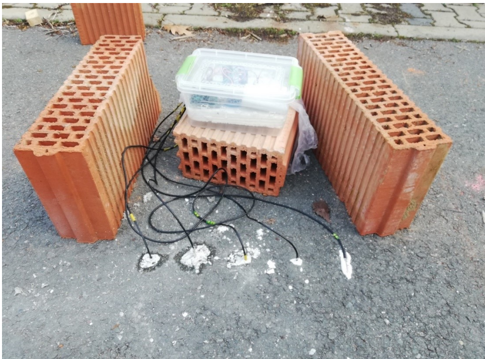
Figure 19 Thermometer sensors installed in the site number 1, flexible pavement
