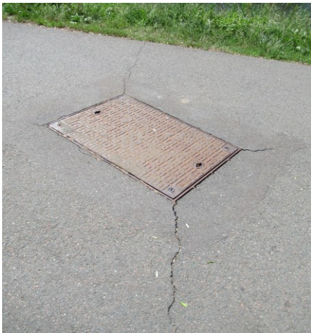
Fig. 8.1. Cracks in a bitumen pavement at the corners of a metal cover, which have arisen due to thermal stresses.
