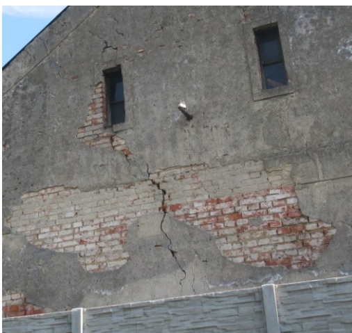
Fig. 9.4. Crack in the wall of an old building
