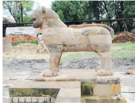
Fig. 17 Patan, a lion at the Bhandarkhal Tank after treatment. (Institute of Conservation, University of Applied Arts Vienna, 2011)
