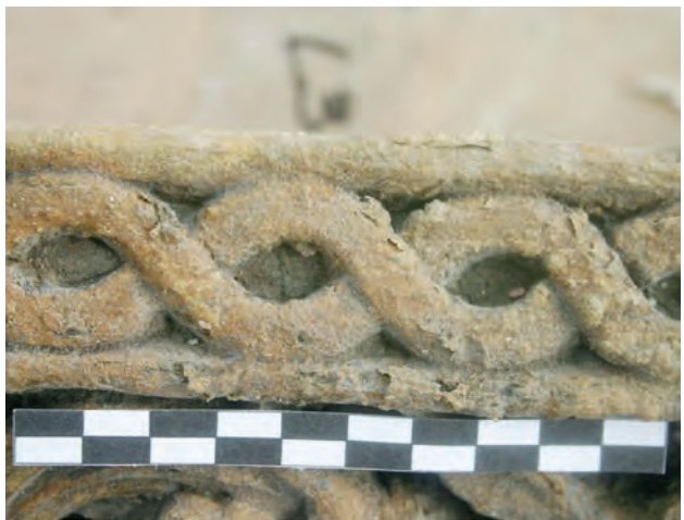
Fig. 5 Patan, Bhandarkhal Tank Pavilion, detachment of the surface and flaking due to a hydrophobic surface coating. (Institute of Conservation, University of Applied Arts Vienna, 2010)
