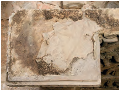
Figure 2 (bottom) Patan, insect nest in one of the joints of the Bhandarkhal Tank Pavilion. (Institute of Conservation, University of Applied Arts Vienna, 2010)
