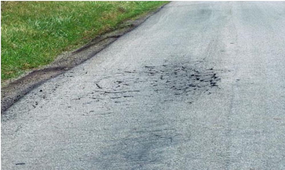
Figure 27: A damaged road by heavy trucks Source: (5)
