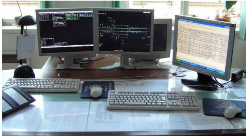
Figure 16: Modern IT for controlling the railway traffic (Station Master, DOZ interlocking)
