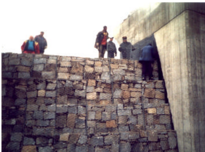
Obr. 3 Kóí dlo mostu z dráokoš ù– gabionù Fig. 3 Wing of bridge from wire-scrapes - gabions
