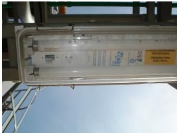
Figure 79 – Oil & Gas – light fixtures
