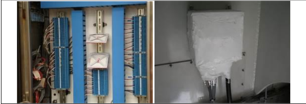
Figure 77 – Oil & Gas – electric panel
