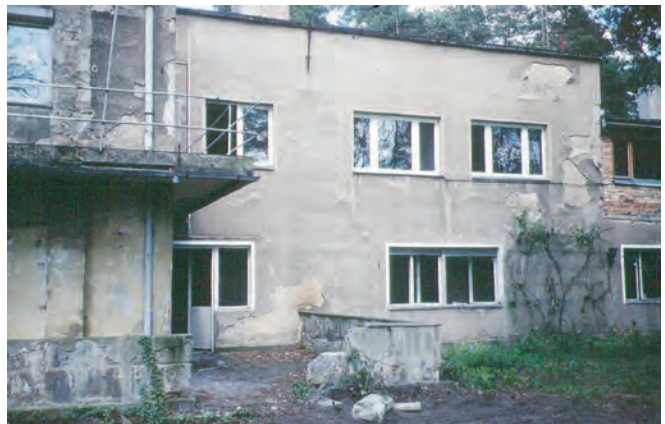
Fig. 8 Masterhouse Muche/ Schlemmer, facades before uncovering of the original plaster, 2002. (Photo Danzł).
