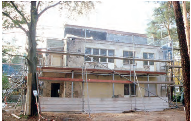
Fig. 7 Masterhouse Kandinsky/ Klee, eastern facades after chopping of the original plaster with conserved "campioni", 1998. (Photo Danzł)
